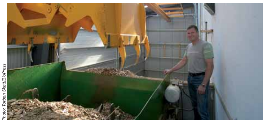
Production manager Torben Brand Andersen at the crane, which supplies wood chips to the vaporizer and the boiler.
